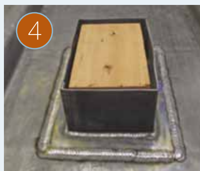
4 Lead slate welded in position. Hot work permits and fire safety precautions should be used.
